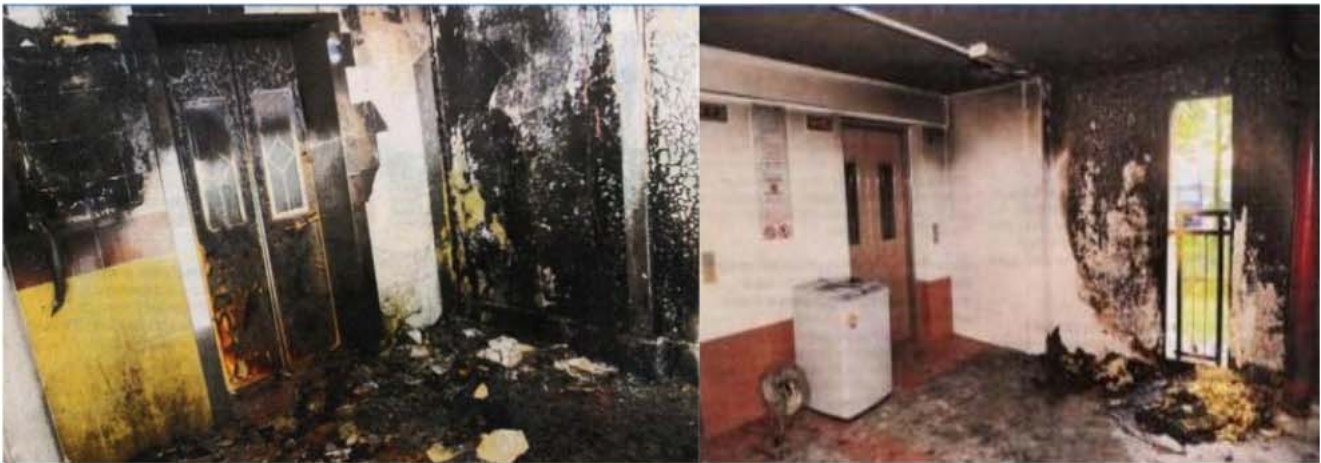
Fire damage to lift lobby involving discarded mattress
