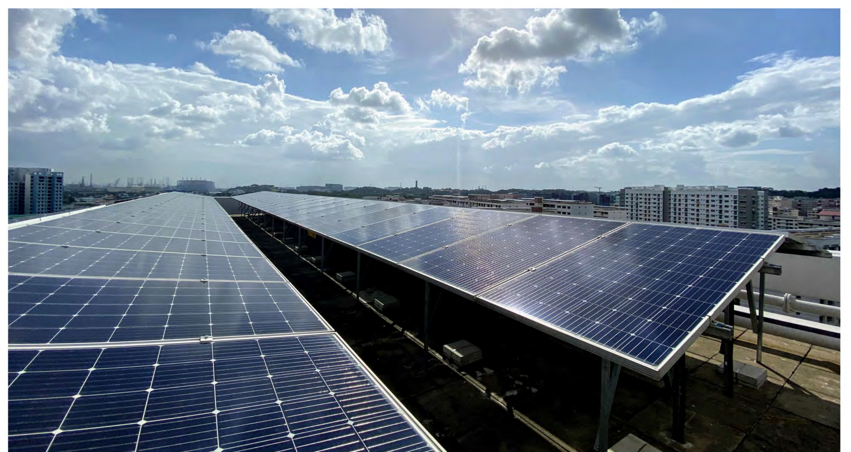
We have installed rooftop solar panels to harness clean energy and promote sustainability
